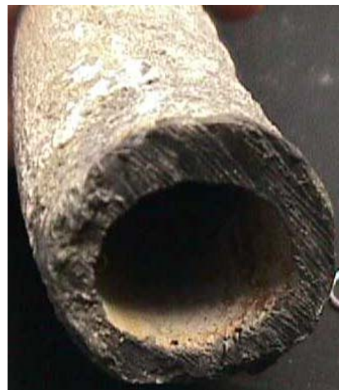
Unsafe, Corroded Lead Pipe
